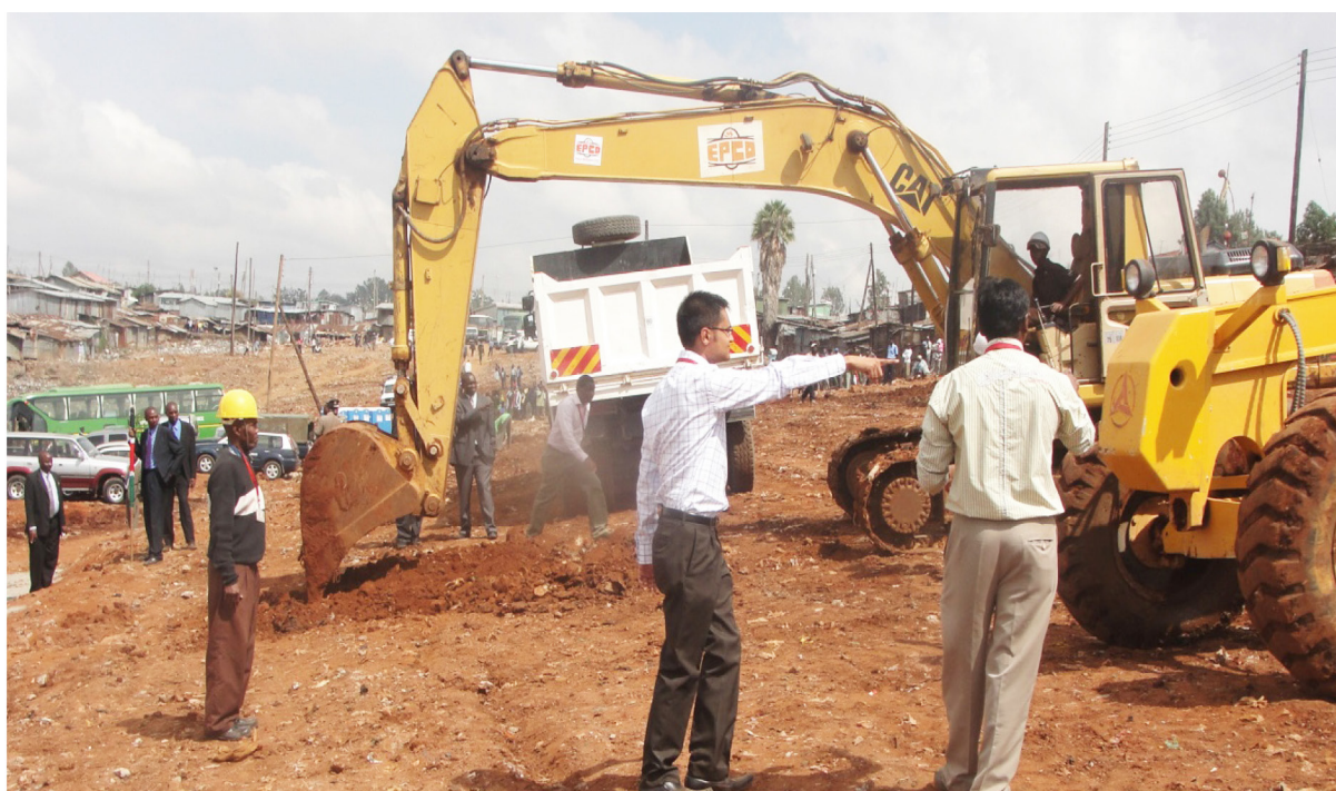
Excavators at work at the Soweto East construction site in Nairobi, one of the KENSUP projects
